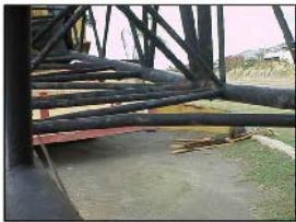
Bent lattice member
