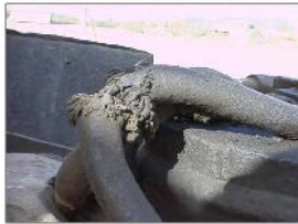
Deteriorated hydraulic hose
